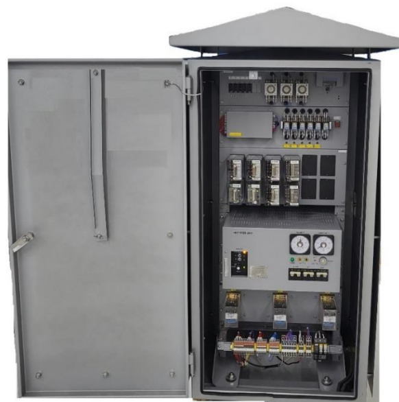
Crossing Control Unit Equipment box
